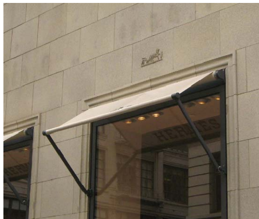
Retractable awnings can be opened for sun protection, and closed when more light is desired.
